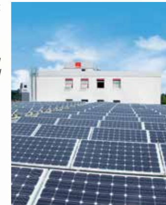
Our contribution to a clean environment is our solar energy roof system
